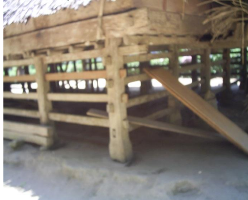
Figure 6. The main pillars of the traditional house in Kaju Bera connected to one another by thin beams called pelelen (Source: Authors' research results).
