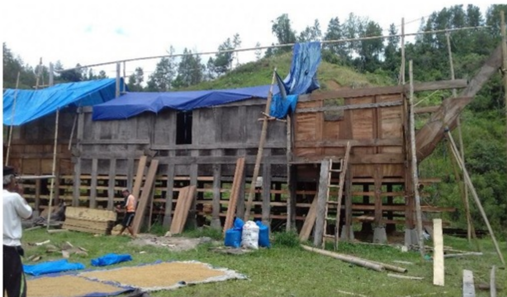
Figure 2. Installation of pole and wall construction has been completed (Banua Sikapu'mi) Source: Research Results
