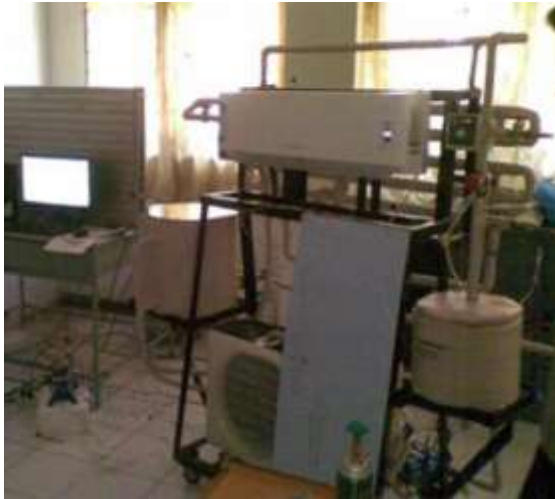
Gambar 3. Instalasi sistem chiller skala laboratorium
